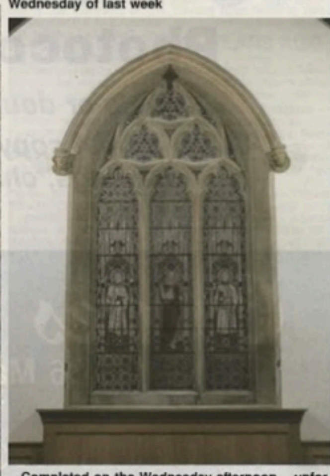
Completed on the Wednesday afternoon – unfortunately the leaden sky with heavy rain meant not much light was shining through!
