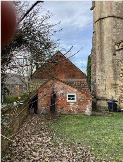
Curfew Cottage - crack to east elevation
