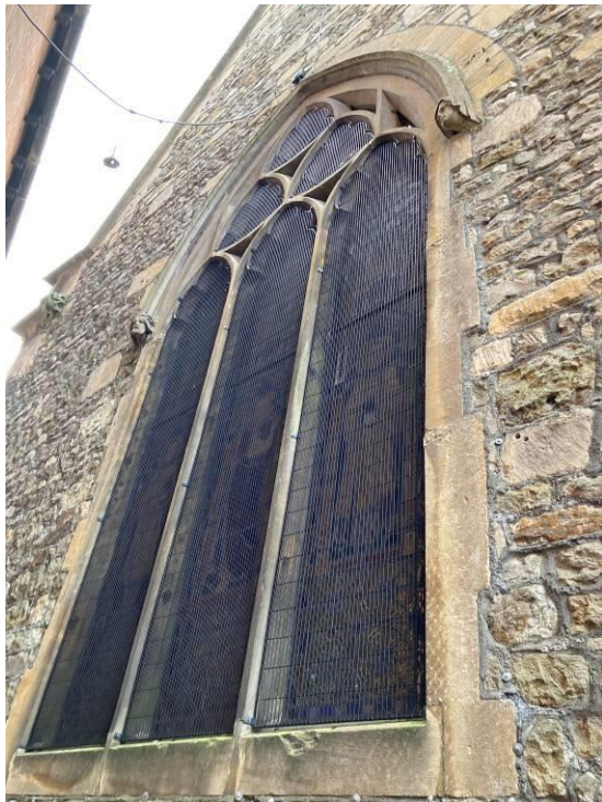
East Window – mesh fixings /cracking to stone sill.
