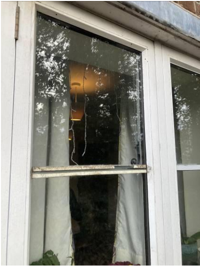
Missing bar detail.
